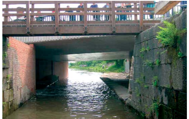
A comprehensive range of bridges are available
